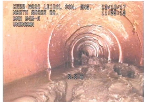
CCTV inspection of storm drain system found considerable sediment build up in some pipes
