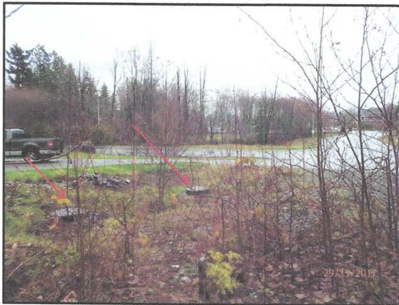
The man-holes (marked with red arrows) of the stormwater infrastructure that is positioned under Point Ideal Road.
