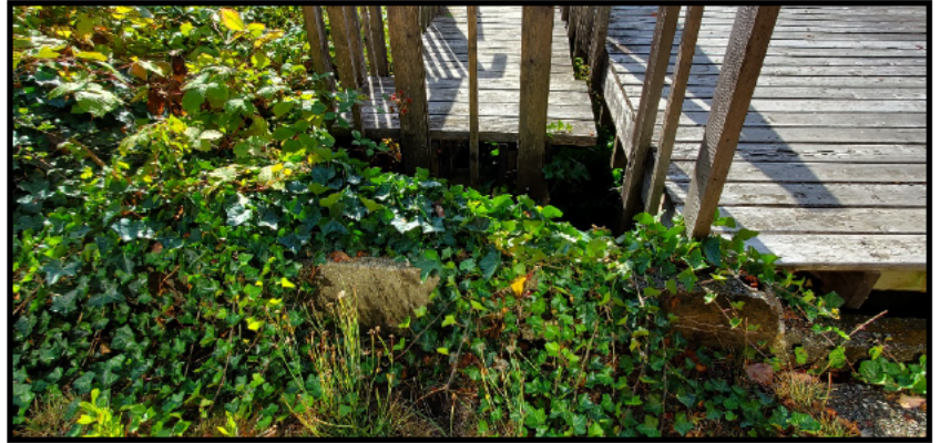
Images (above & Left) Vegetation at top of retaining wall predominately English Ivy, blackberry and hardhack. Area dominated by Invasives.
