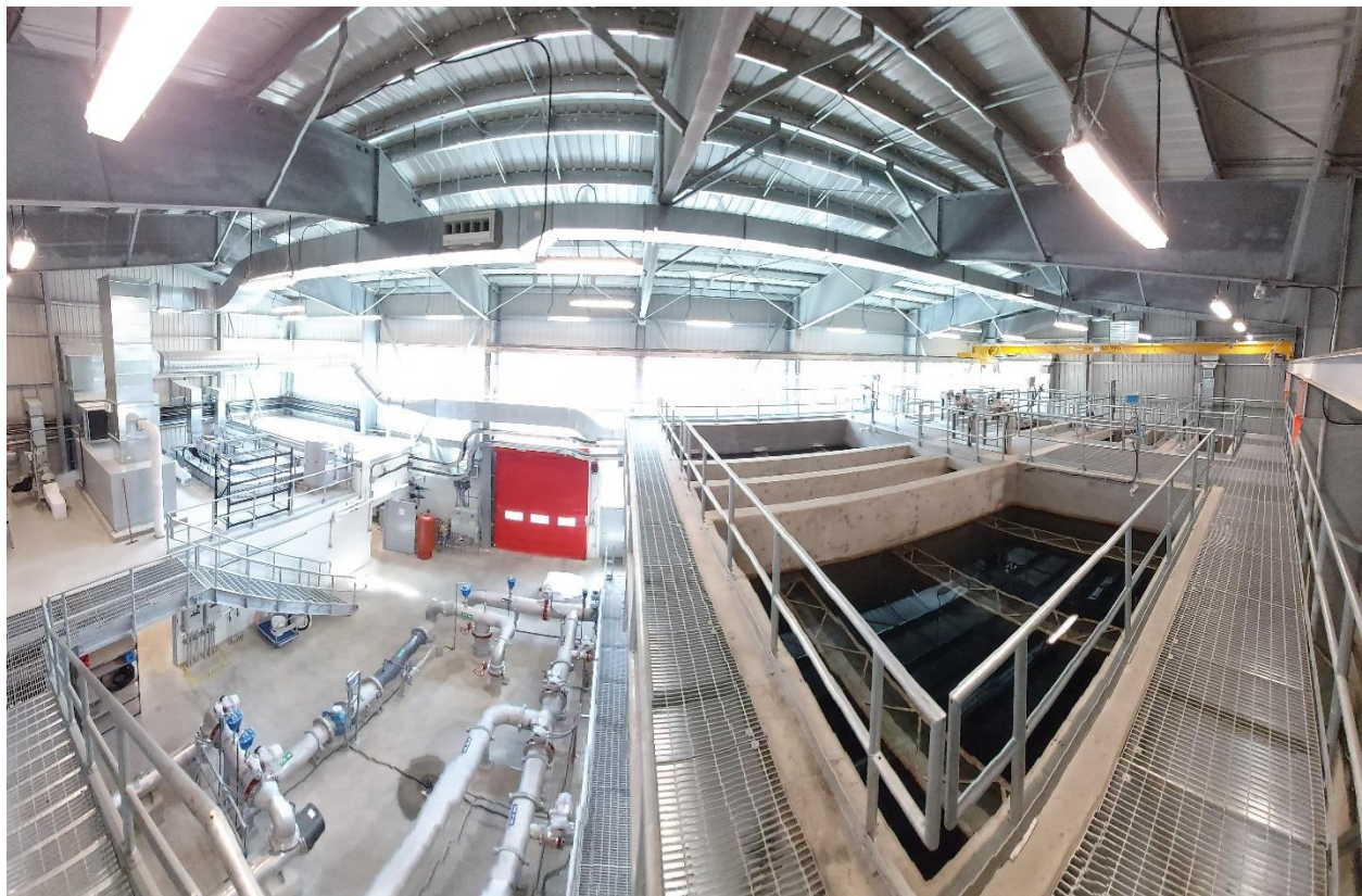
Interior panoramic showing (from right to left) the HVAC system, pipe gallery with UV disinfection system, anthracite/sand media filters, flocculation tanks.
