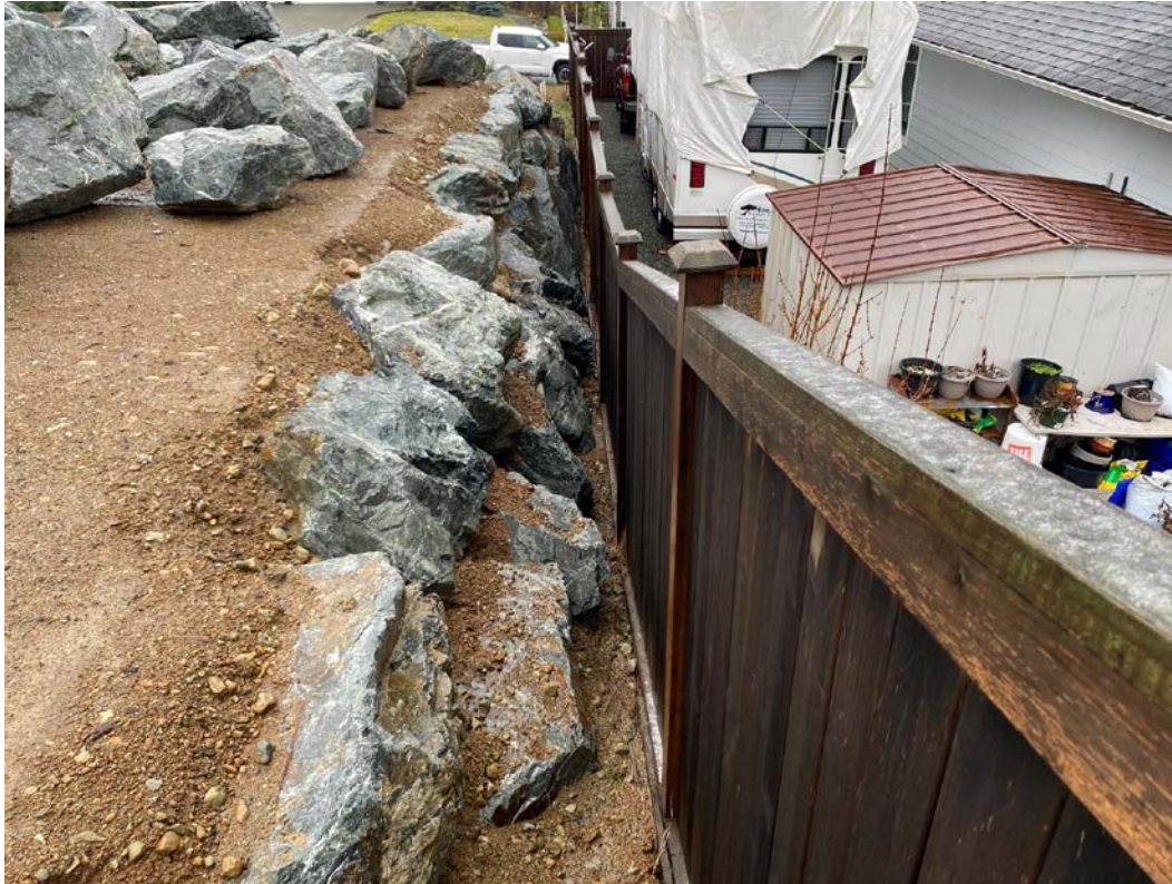
Figure 2.4.3 – West Property boundary showing 1.8m stacked rock wall and fill above, looking south.
