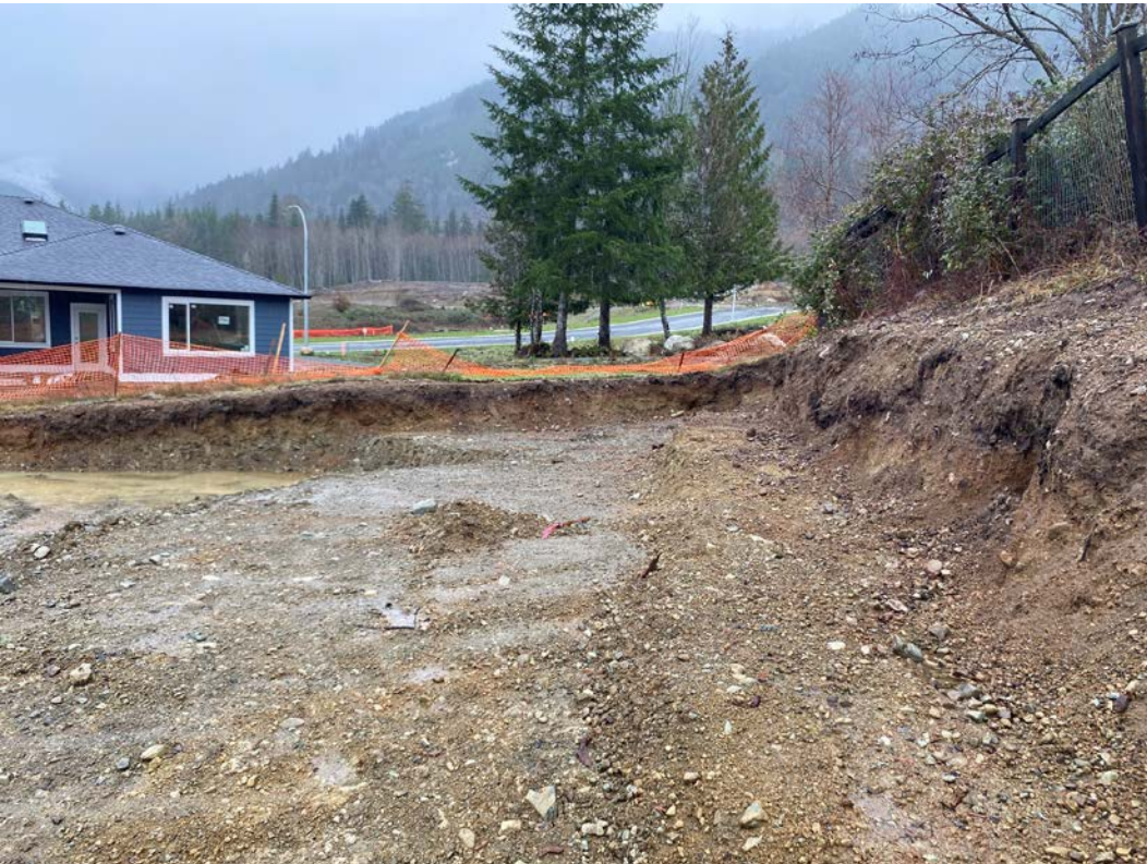
Figure 2.4.2 – Rear of Property showing existing excavations to dense till soils, looking north.
