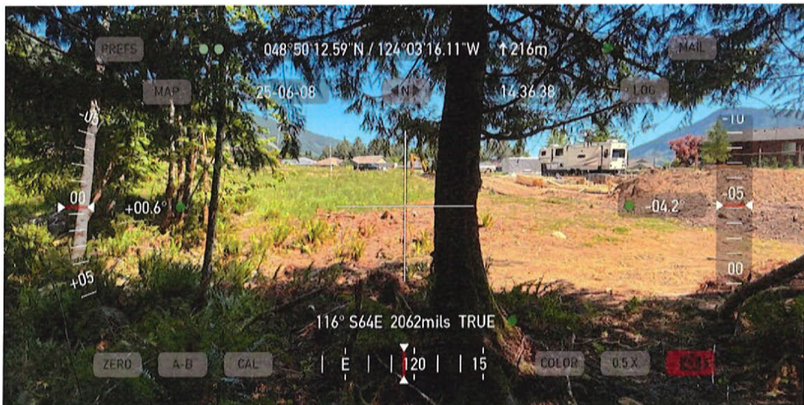
Looking from forest edge (outside of SPEA) (in RAA) toward house site. Lot 1(right) non-riparian under house construction.
