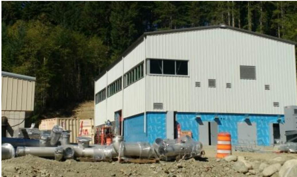
Figure 16 Water Treatment Facility on Indian Road
